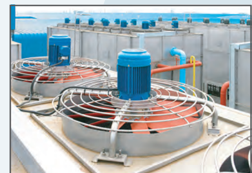
Fan and water pump
